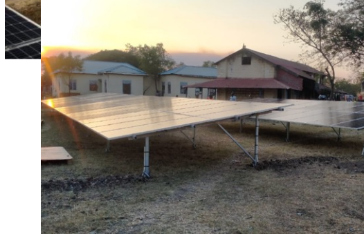
Hospital solar electrification
